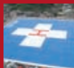
ALUMINUM HELIPORT Uwajima City Hospital
